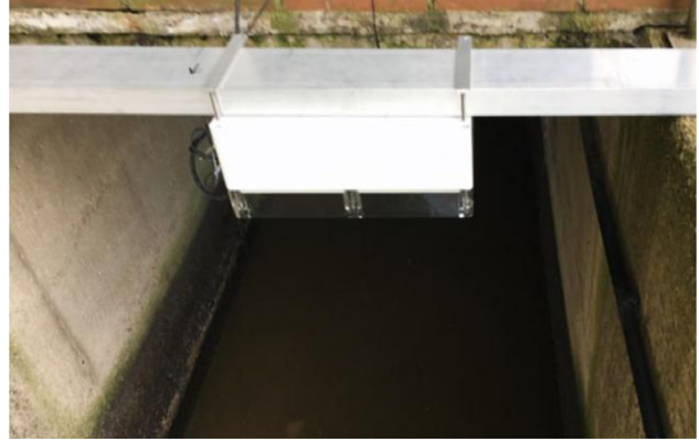
Fig. 2. Placement of the recording hardware into an open channel.
